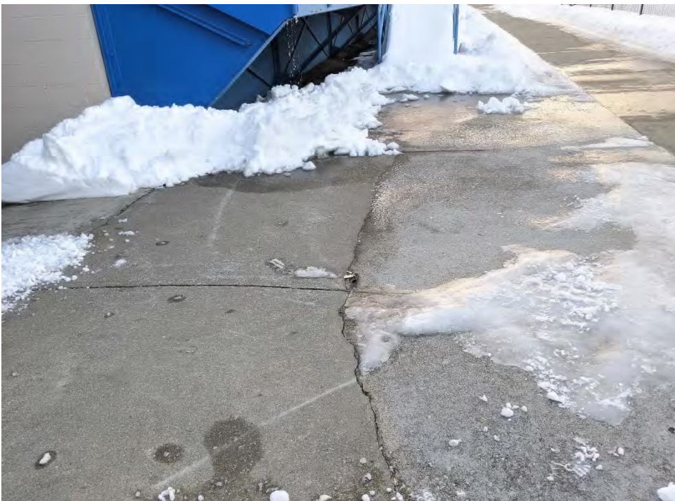
Photo No. 6: Existing crack near the entrance of the stadium
