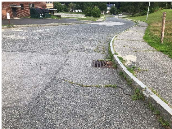
Picture 2: Pavement Deterioration East Access Drive
