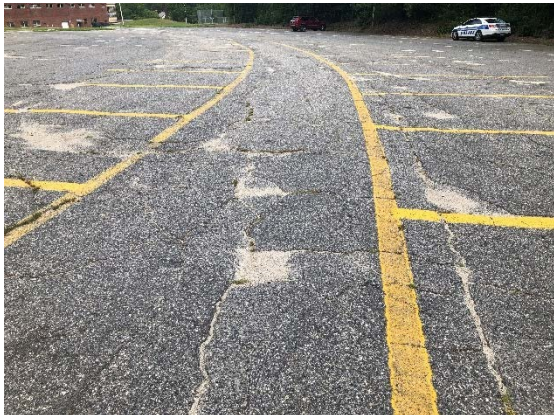
Picture 1: Pavement Deterioration Upper Parking Lot
