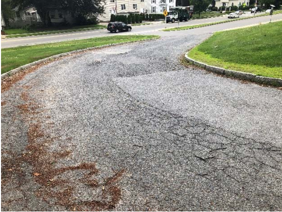
Picture 5: Pavement Deterioration Service Area Access Drive
