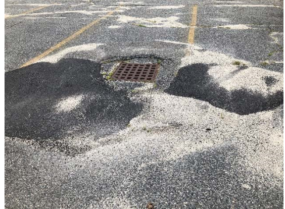
Picture 6: Pavement Deterioration East Parking Lot
