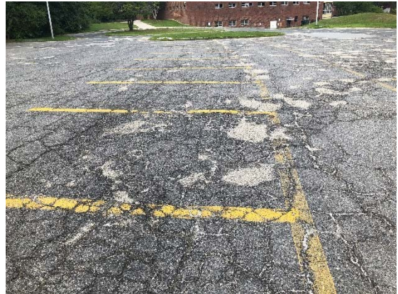
Picture 3: Pavement Deterioration Upper Parking Lot
