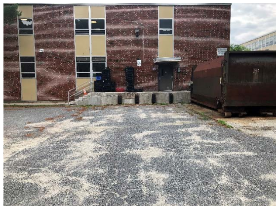
Picture 4: Pavement Deterioration Service / Loading Area
