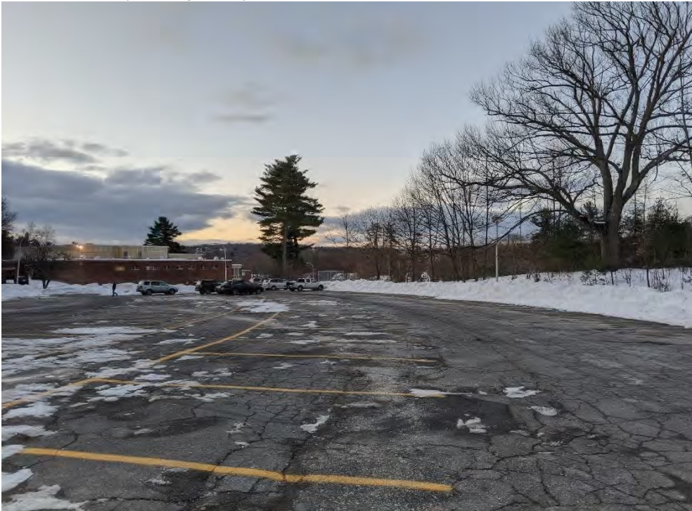
Photo No. 2: Asphalt condition in the existing parking lot to the existing building
